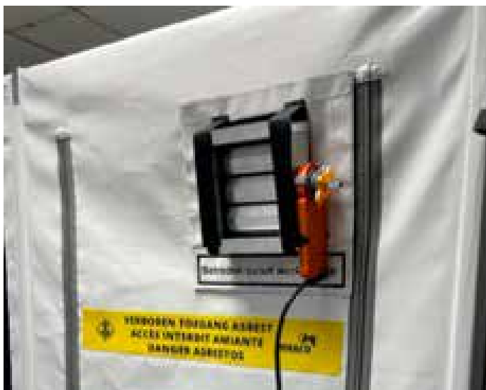
Figuur 4 Opening Dehaco Bypass
